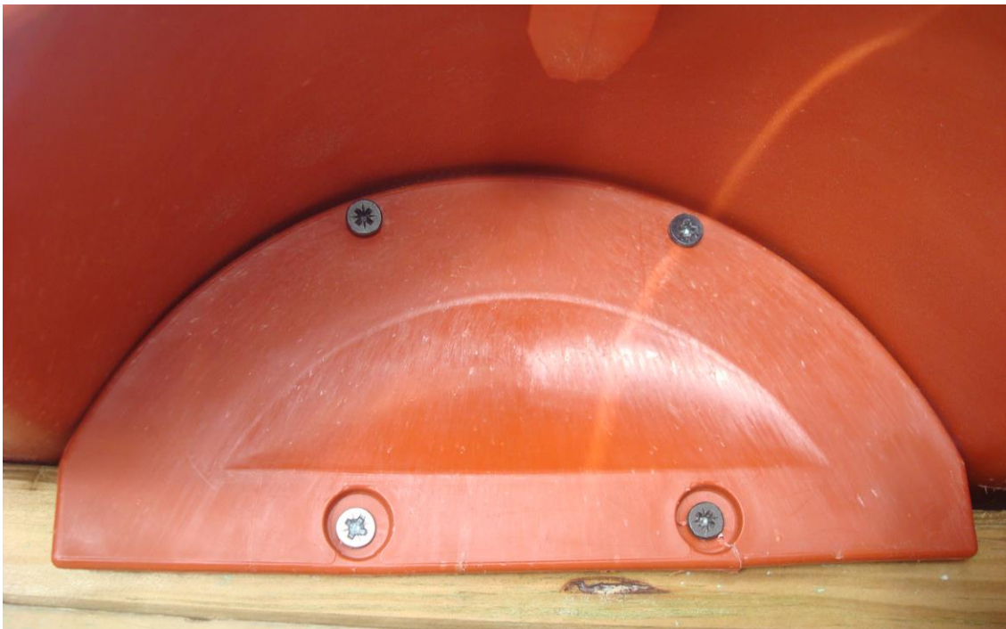
Picture of the installed anti-bird closure
